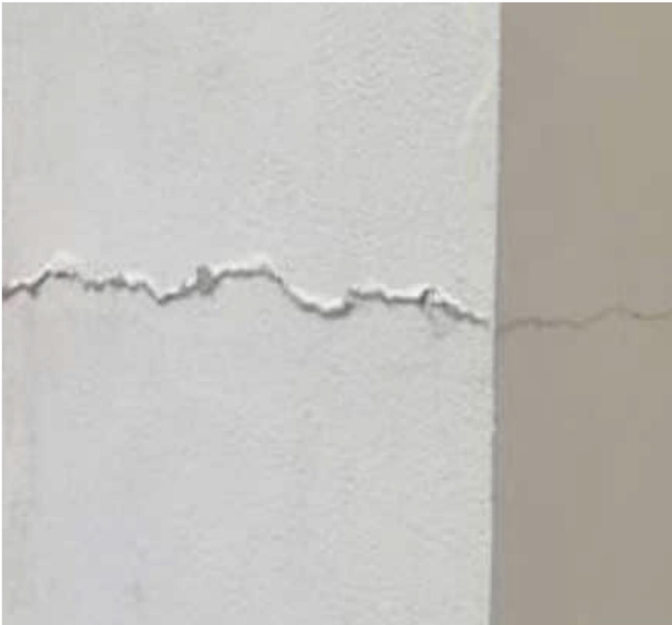
Cracking due to thermal movement
