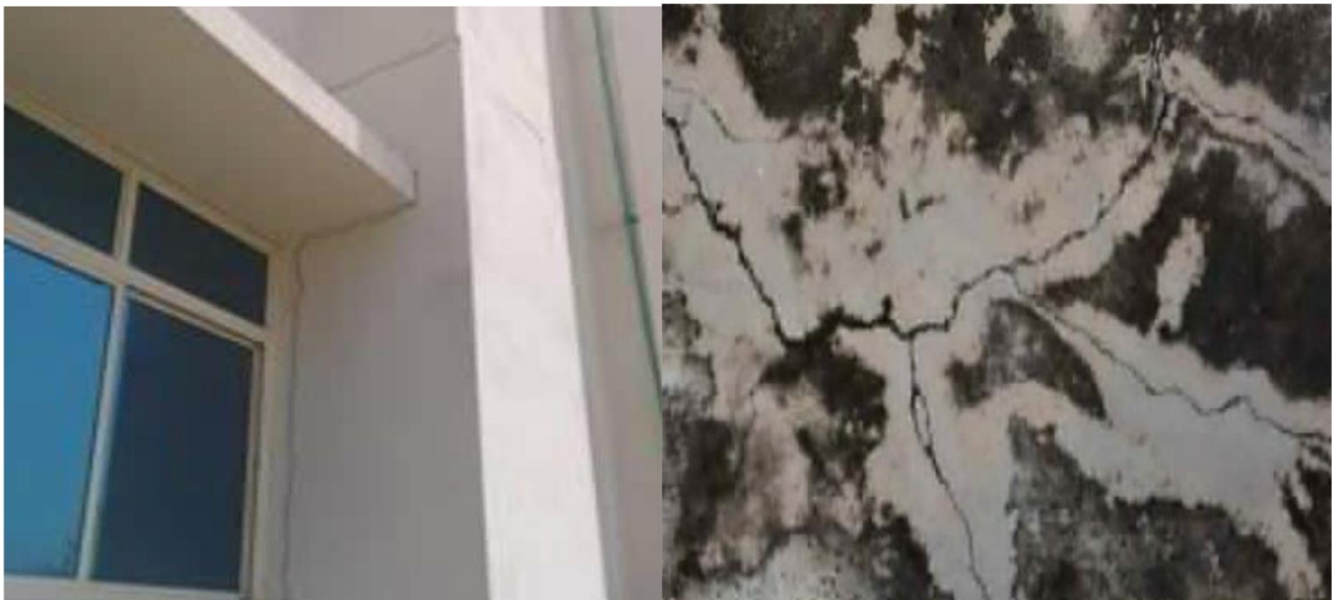
Crack above window due shrinkage
